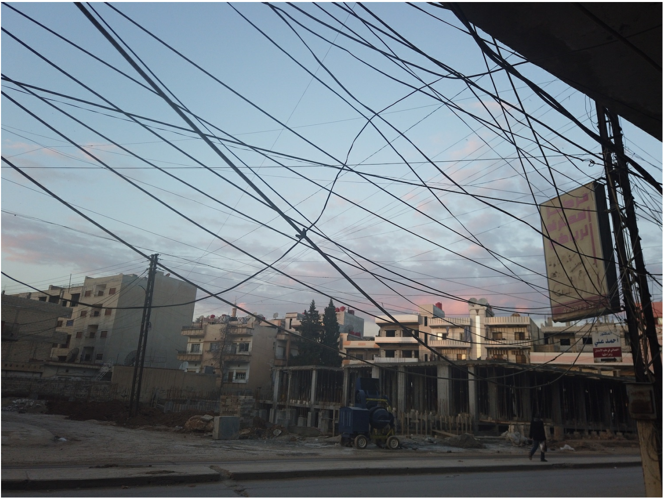
Electricity cables in Qamishli, Northern Syria
